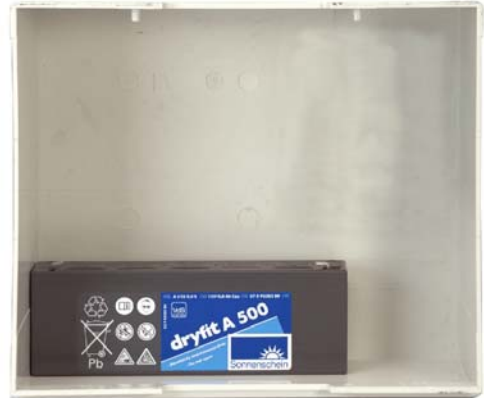
Cover with installed battery
